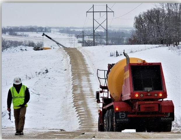
Application of a beet juice-chloride blended deicing solution to snow covered wooden
