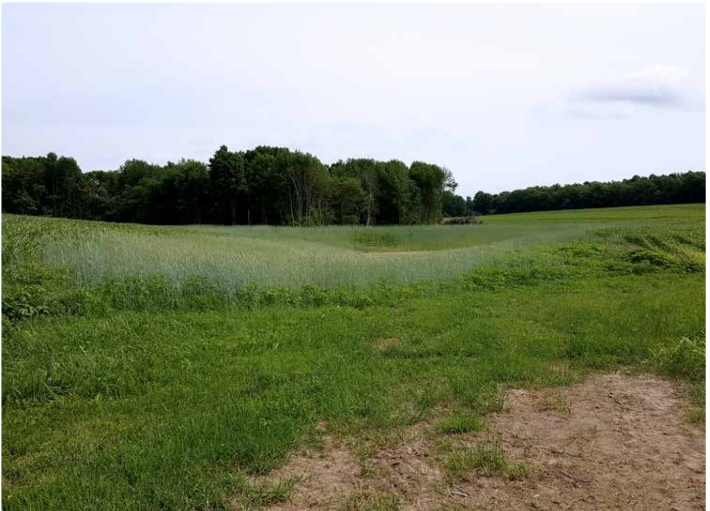
Grade stabilization structure site the spring following construction. Photos courtesy of Dunn County.
