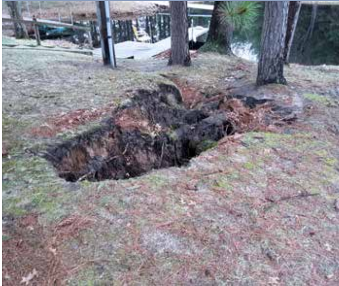
Large hole in the bank of Arnold Creek near Lake Arbutus. Photo courtesy of Clark County.
