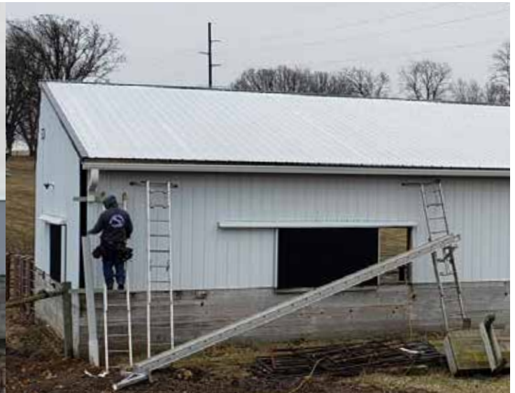
AFTER - Installing roof gutters at the Laeser property. Photo courtesy of Iowa County
