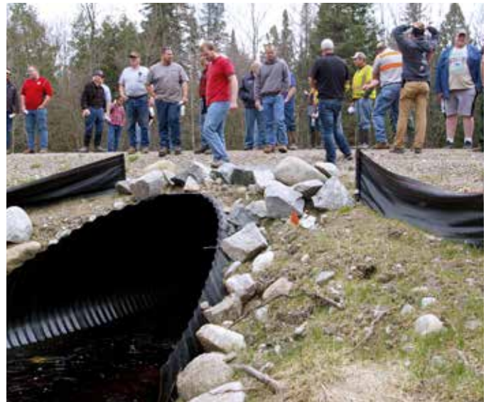
Tour of newly constructed stream crossing in Forest County. Photo courtesy of Forest County.
