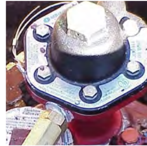
Mechanical Line Leak Detector
