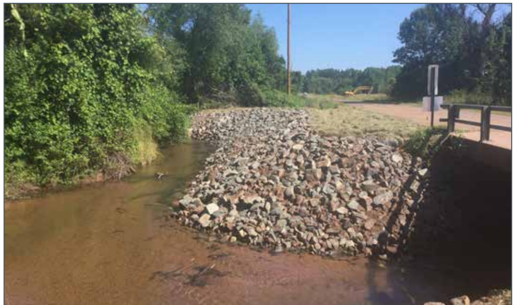
The completed streambank riprap installed on Whittlesey Creek reduces sedimentation and protects the stream crossing
