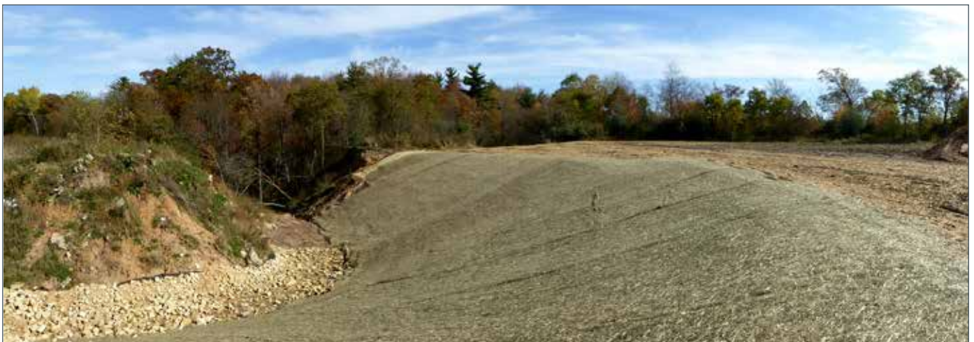
Finished project: Rock-lined channel and seeded slopes protected with erosion control mats
