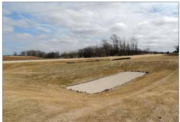
Completed iron filtration bed on the north edge of Jen's property (looking north towards the lake)
