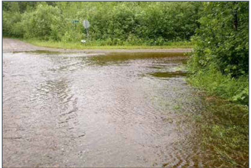
Significant 2017 rains and an undersized culvert led to flooding
