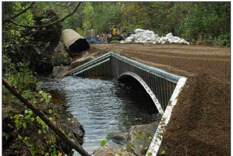
The new culvert has a higher capacity. The old undersized culvert can be seen in the background
