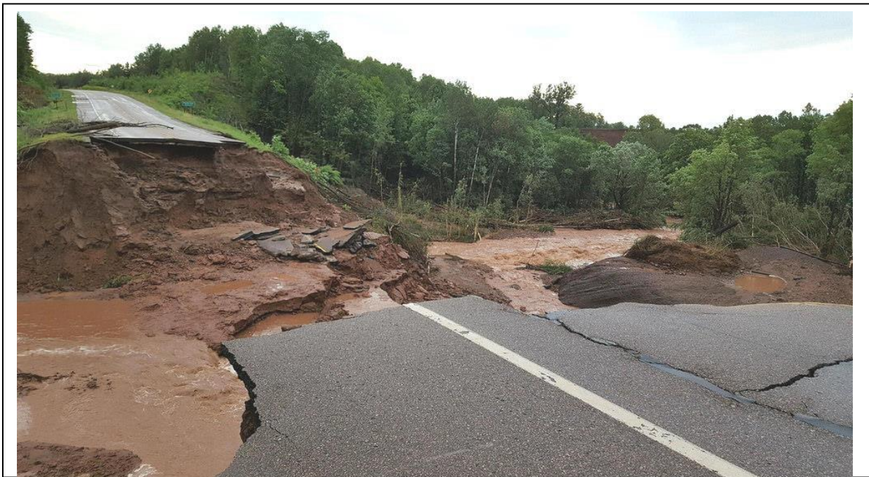
State Highway 13 at Highbridge, WI. Ashland County. Wisconsin Emergency Management, July 13, 2016
