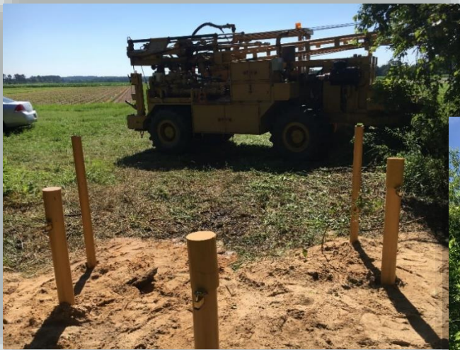
Left: Sun setting on a job well-done: three new monitoring wells with protective bumper posts installed next to a potato field.
