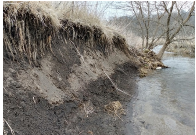
Steep streambank erosion, Ridgeway, WI
