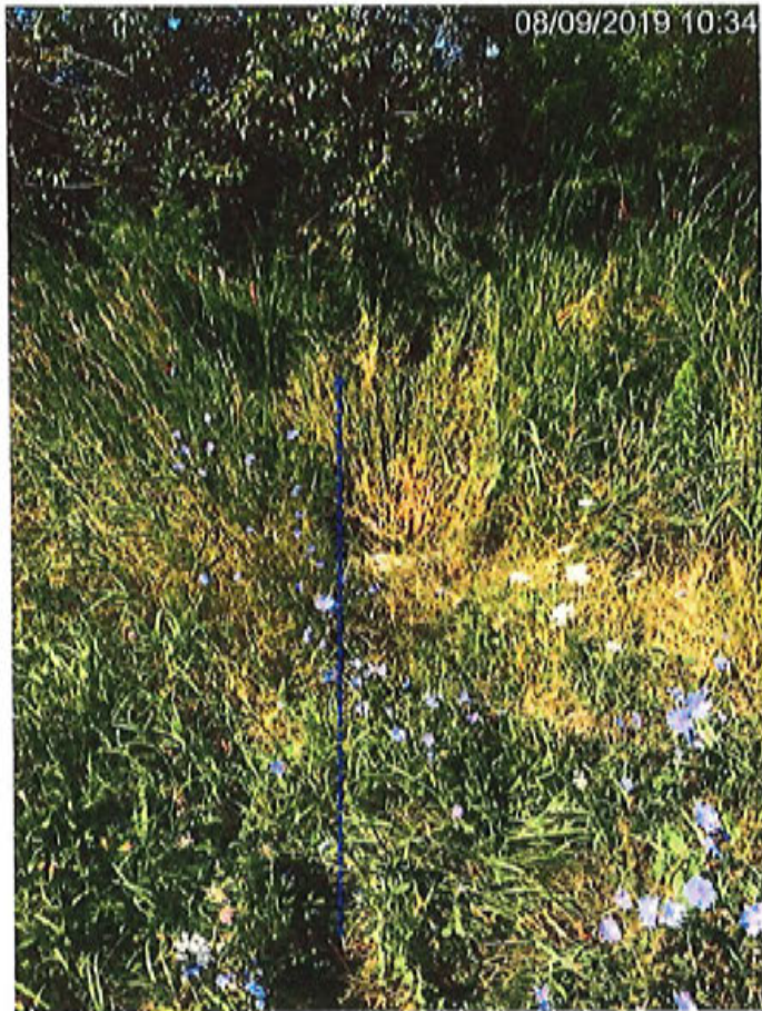
Photo 7 (left). West side of Chestnut Drive at road culvert (facing west). Blue arrow indicates the direction of flow from the road culvert.
