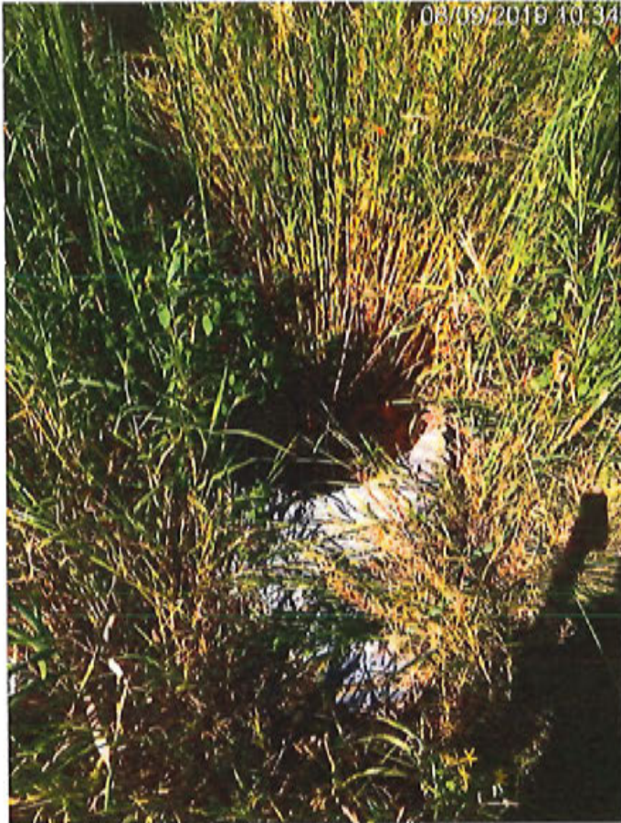
Photo 5 (left). Road culvert on west side of Chestnut Drive, north of N7574 Chestnut Drive.
