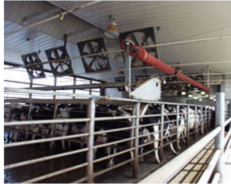
Crowd gates may not use much electricity; however, proper installation and maintenance help insure against possible transient stray voltage problems. -- Photo Karl Ohm
