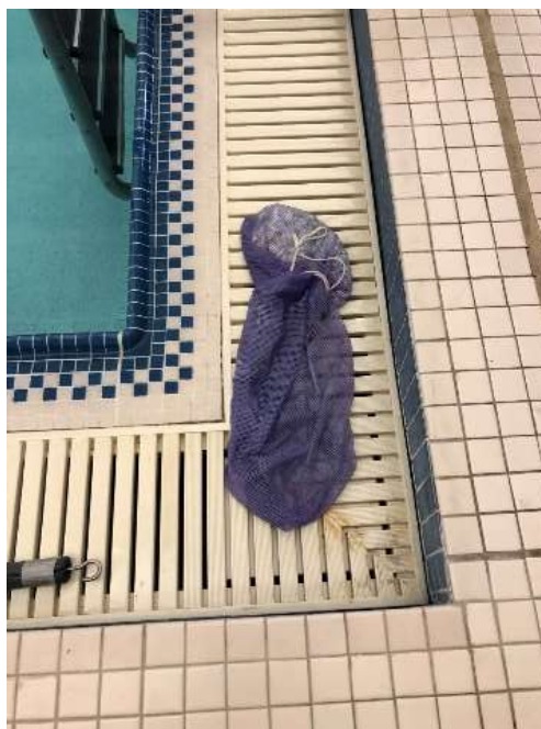
Figure 3b. Placing chemicals in skimmers or gutters is not an approved method of adding chemicals to the pool.
