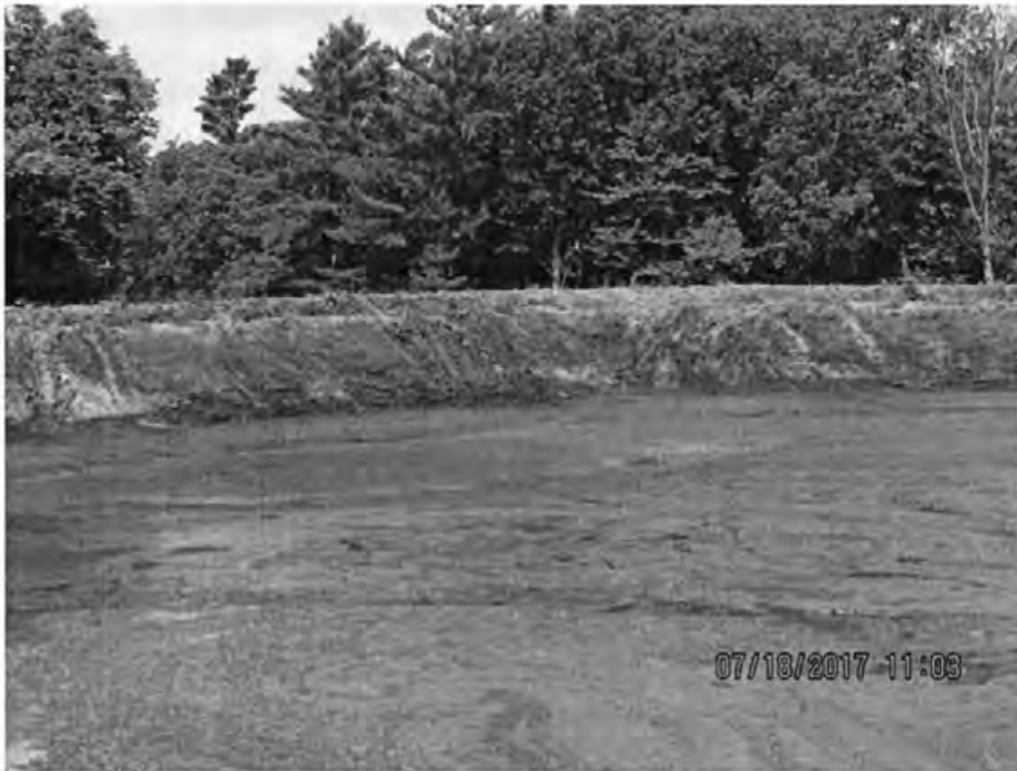
Photo 32: Close up view of the interior western wall of outfall/WSF 001. Photo direction is west.
