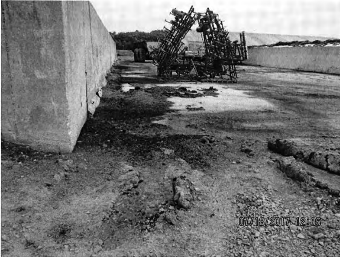
Photo 75: View of a concrete wall from the middle of the feed storage area at the heifer site. Leachate was observed discharging from the wall (black liquid/substance). Photo direction is east.
