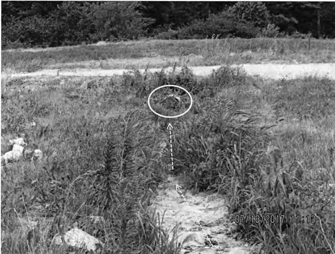
Photo 49: Close up view of the culvert through which storm water flows on the east side of the main farm in front of the freestall barn and milking parlor. Yellow dashed arrows indicate direction of flow path. Yellow circle is the culvert. Photo direction is north.
