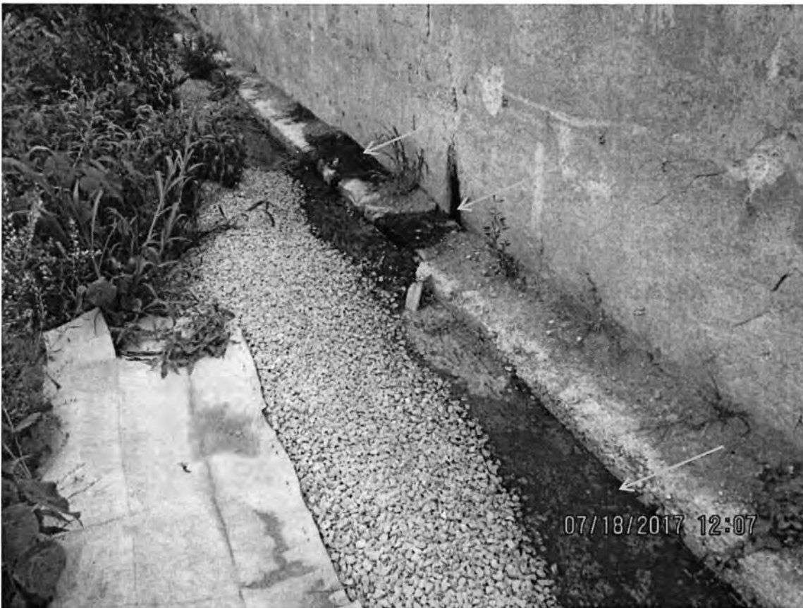
Photo 76: Close up view of the concrete wall on the NW side of the feed storage area at the heifer site. Leachate was observed discharging from the wall and was ponded adjacent to the wall (orange arrows). Photo direction is NE and down.
