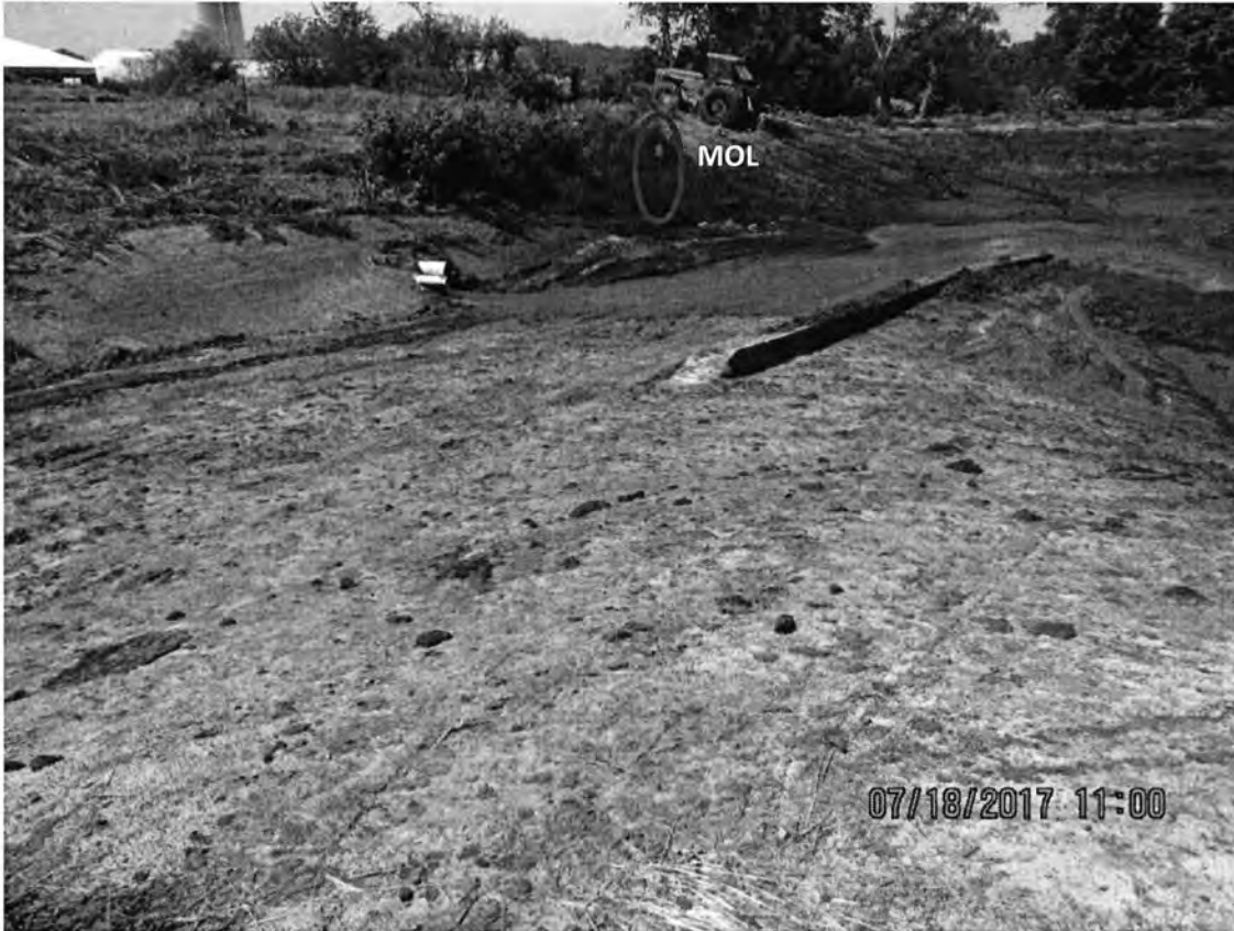
Photo 26: View of the southern section of outfall/WSF 001 showing the concrete ramp. Photo direction is west.
