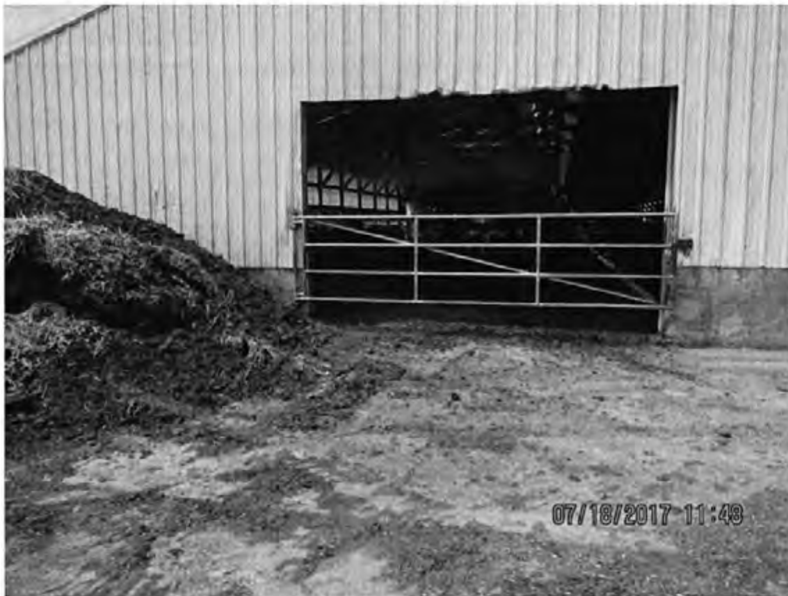
Photo 11: Close up view of the east end of the heifer/calf barn. Photo direction is west.
