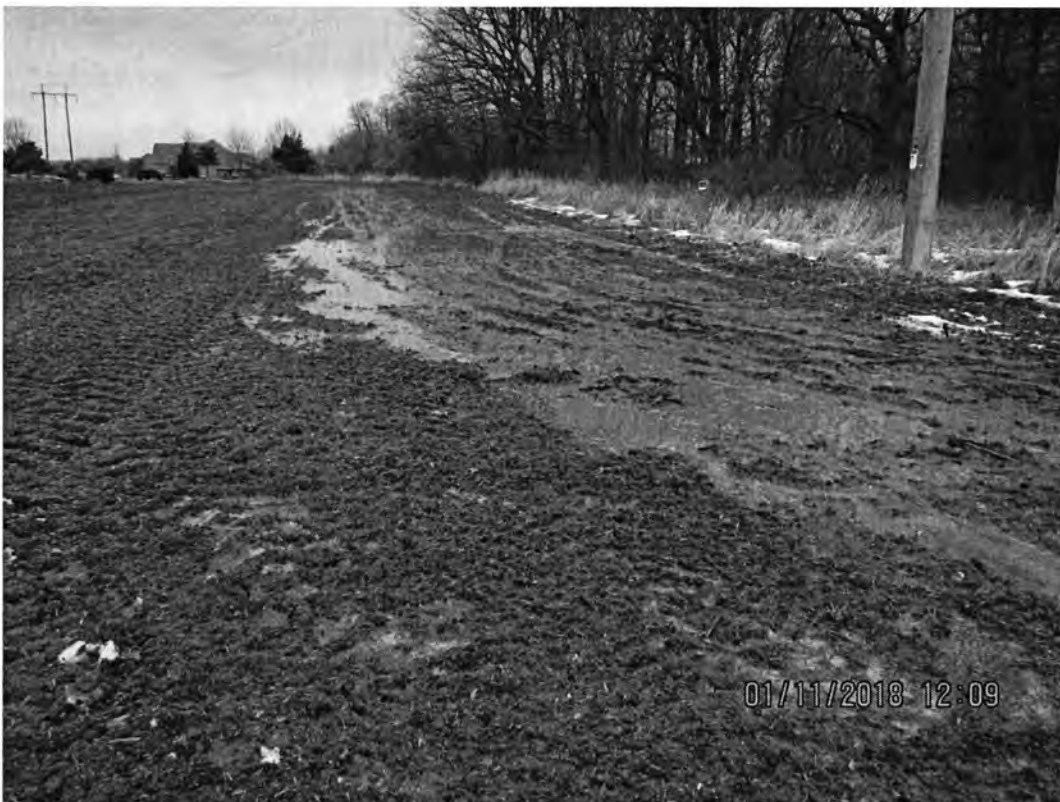
Photo 14: View of the NE corner of 11L-East showing ponded storm water from snowmelt. Photo direction is north.
