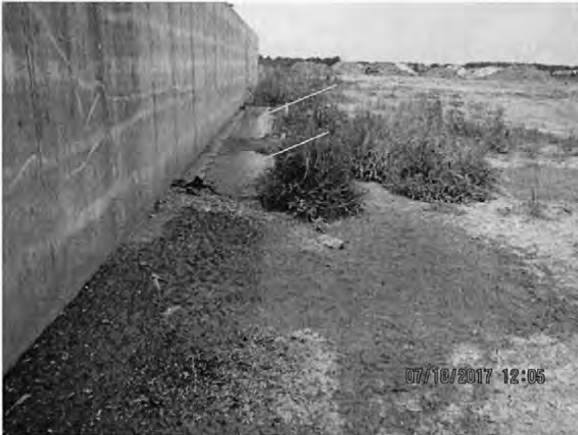
Photo 73: Close up view of a concrete wall from the middle of the feed storage area at the heifer site. Ponded leachate was observed adjacent to the wall (orange arrows). Photo direction is west.
