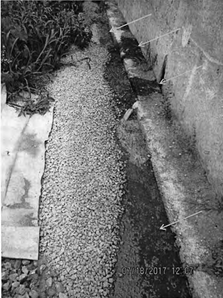
Photo 77: Alternate view of the concrete wall on the NW side of the feed storage area at the heifer site. Leachate was observed discharging from the wall and was ponded adjacent to the wall (orange arrows). Photo direction is NE and down.
