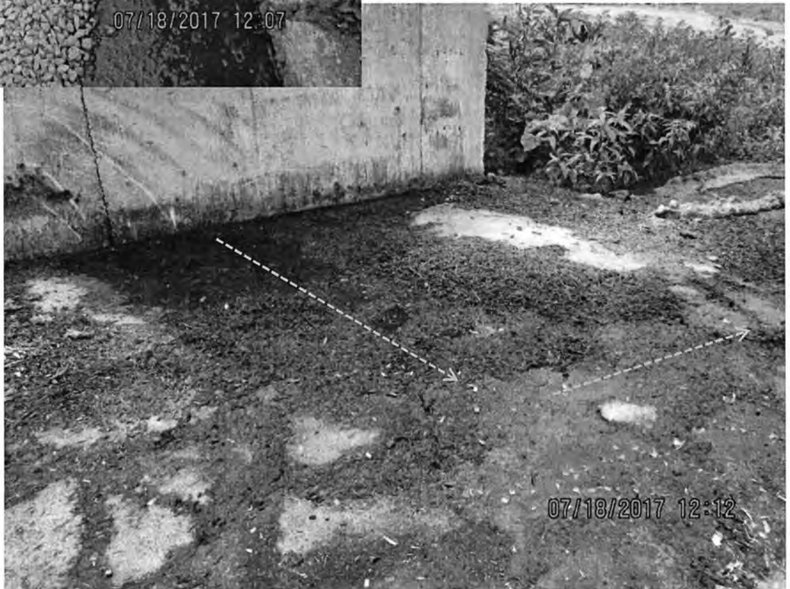
Photo 78: View of the north concrete wall of the feed storage area at the heifer site. Leachate was observed discharging from the wall. Orange dashed arrows indicate flow path of leachate discharge. Photo direction is SW and down.
