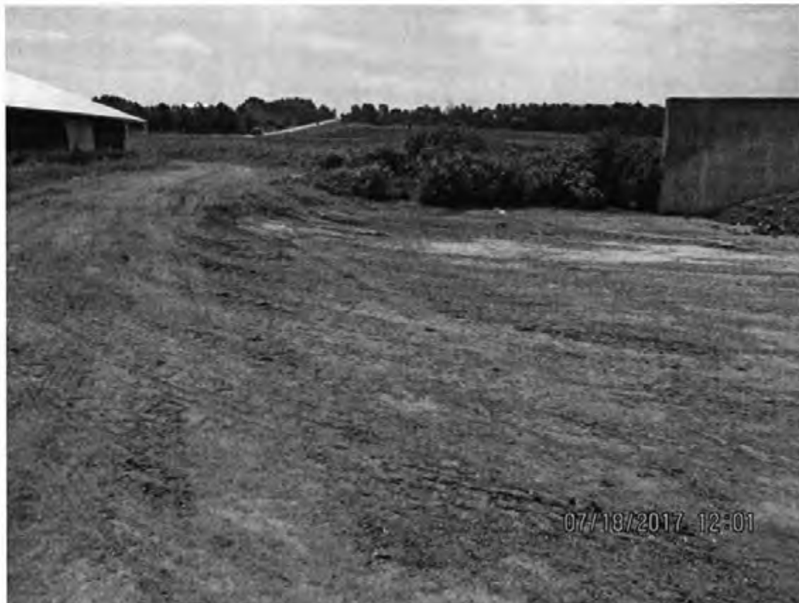
Photo 70: View of the area adjacent to the south wall of the feed storage area at the heifer site. Photo direction is south.
