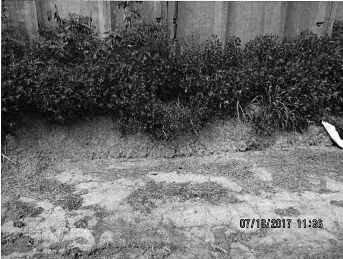
Photo 42: Close up view of the east wall of the feed storage area at the main farm site showing clay placed along the bottom of the wall to prevent leachate discharges. Photo direction is west and down.
