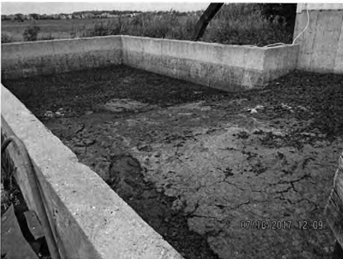
Photo 65: View of outfall/WSF 002 at the heifer site. Photo direction is NW.
