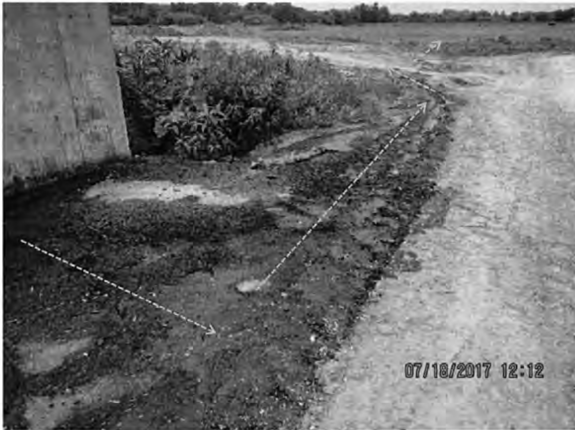
Photo 79: Alternate view of the north concrete wall of the feed storage area at the heifer site. Leachate was observed discharging from the wall and flowing west. Orange dashed arrows indicate flow path of leachate discharge. Photo direction is west.
