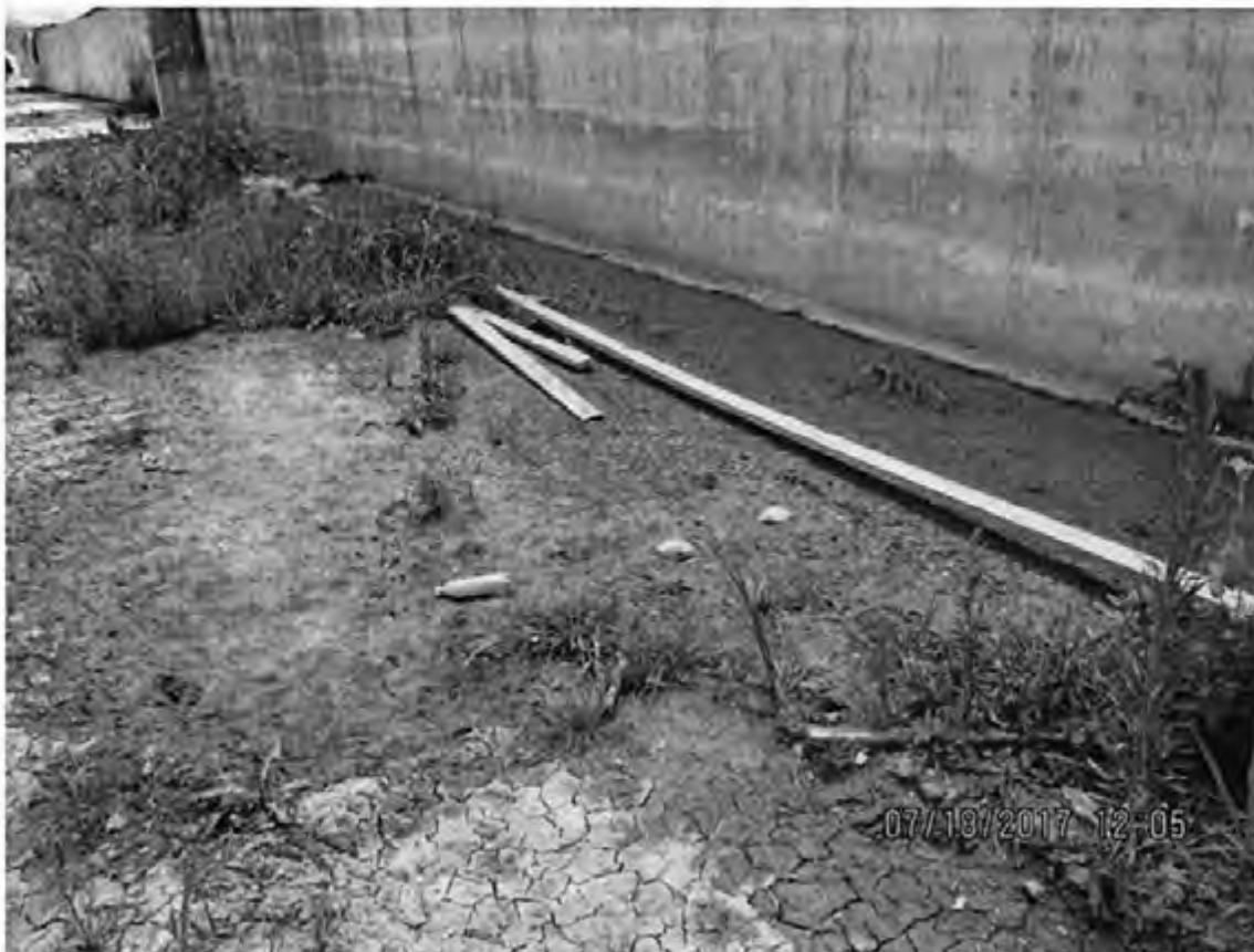
Photo 74: Close up view of a concrete wall from the middle of the feed storage area at the heifer site. Ponded leachate was observed adjacent to the wall. Photo direction is west.
