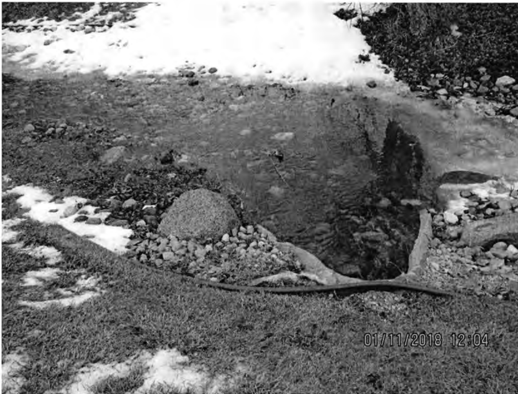
Photo 13: View of the culvert north of Copper Ln where snowmelt discharged from field 11L1. Photo direction is down and north.
