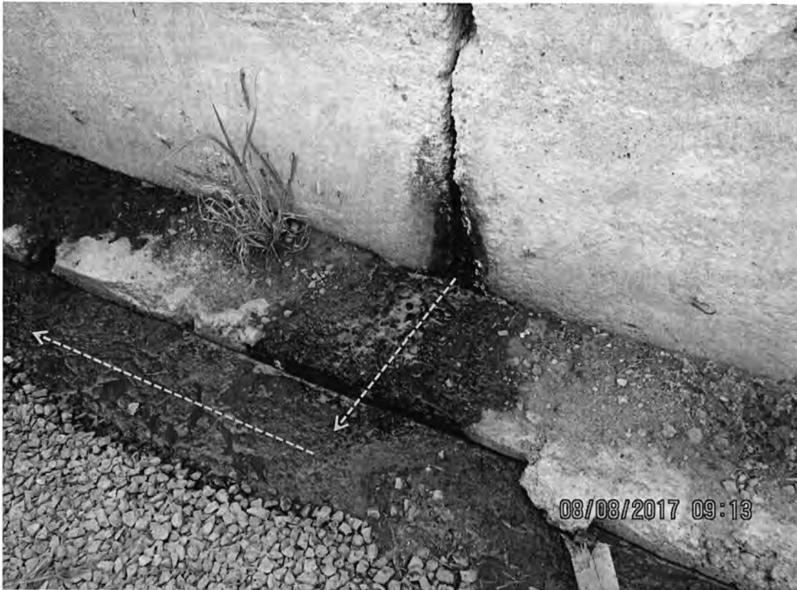
Photo 1: View of a discharge point of leachate / process wastewater on the outer west wall of the feed storage bunker at the heifer site. Dashed orange arrows indicate the direction of discharge flow. Photo direction is down.
