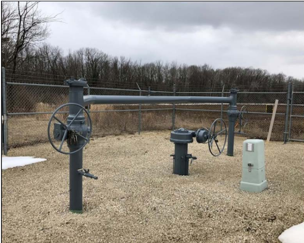
Figure 6: Typical Valve Assembly Facility
