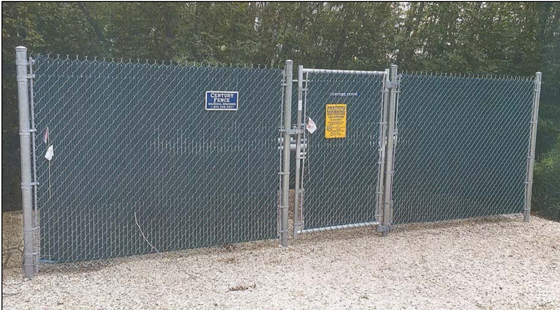
Figure 5: Typical Gate Surrounding Aboveground Facilities
