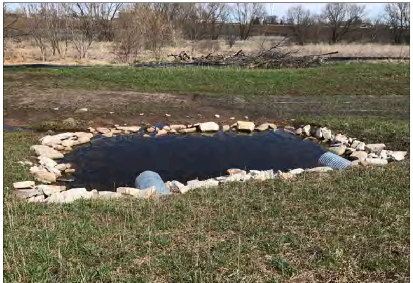
Plunge pool, outletting to a grassed waterway and ultimately a rock lined waterway down slope.
